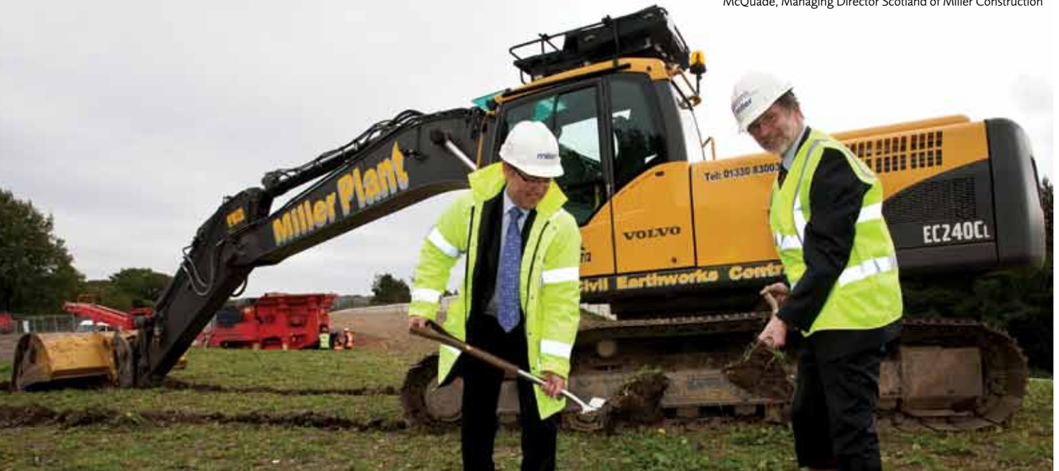
Professor von Prondzynski cuts the first sod assisted by Brian McQuade, Managing Director Scotland of Miller Construction
